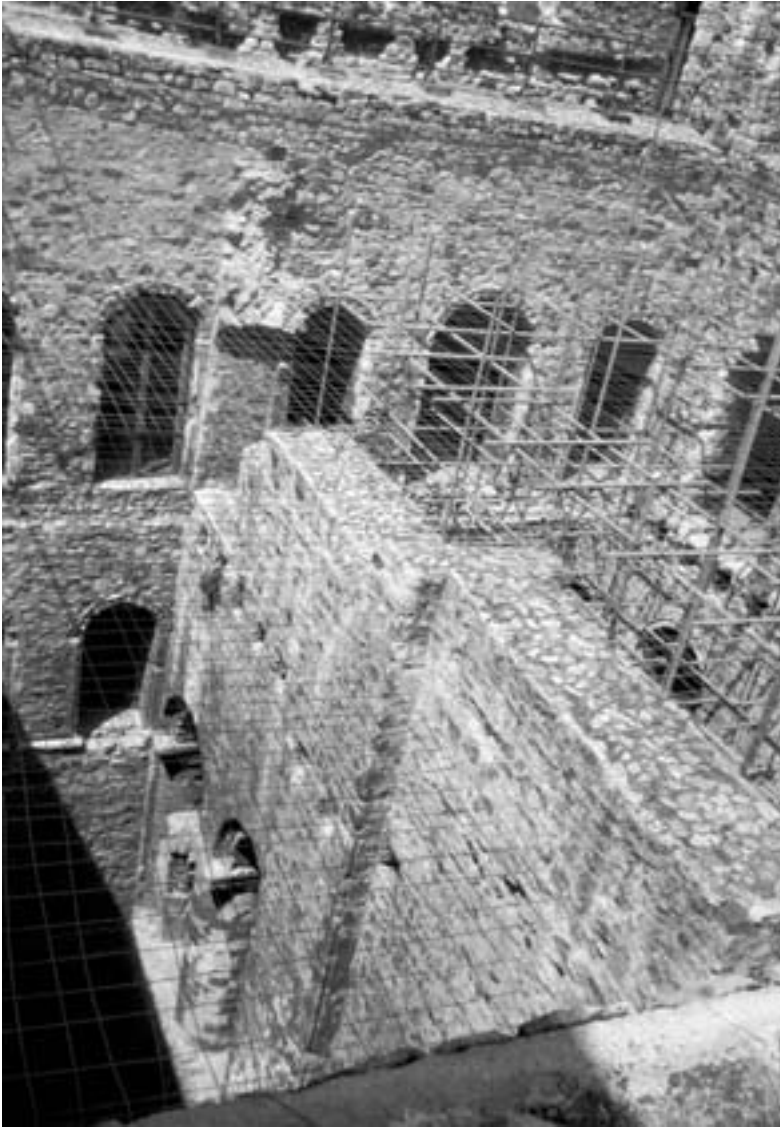
Figure 7. Great tower, Rochester Castle, England, interior. Seen from the top of the wall, the interior stonework of the castle lies exposed. A masonry wall divided the building into two sections. The arches and piers of the principal hall can be seen at the lower left, and the holes for the beams supporting the wooden floors cross the wall at a higher level. Photograph: Marilyn Stokstad.
