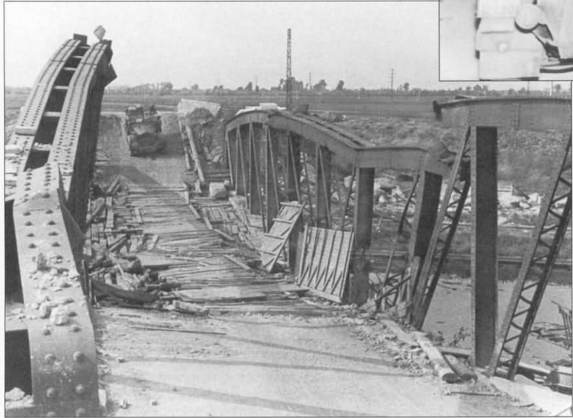
A Kfz.15 medium passenger car approaching a bridge in the Maastricht area, which has sustained considerable damage. This vehicle is part of Hoepner's XVI.Panzerkorps and the photograph was taken during the first day of the invasion. A large unidentified marking appears on the right fender.
