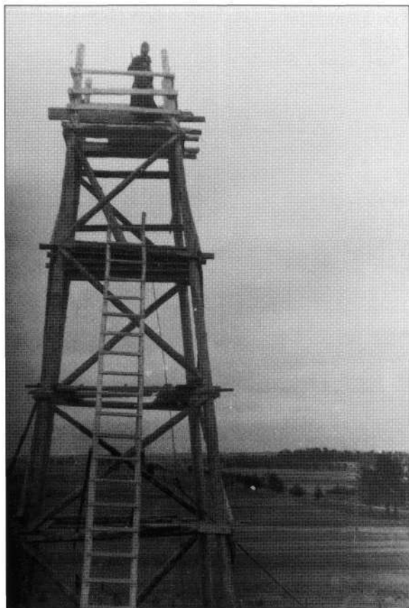
A wooden watch tower being built to overlook Russian positions far to the east. These towers were built during the German advance, but never during the retreat. They were rarely built in the open like this one; rather they were installed at the edges of woods and inside tall trees for camouflage.
