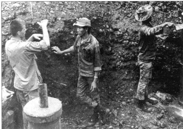
An SF engineer NCO discusses the construction of a below-ground bunker with a Striker, Cung Son, A-221, 1969. Between combat operations, A-team members spent long hours working with the Strikers on camp construction and endless refurbishing projects.
