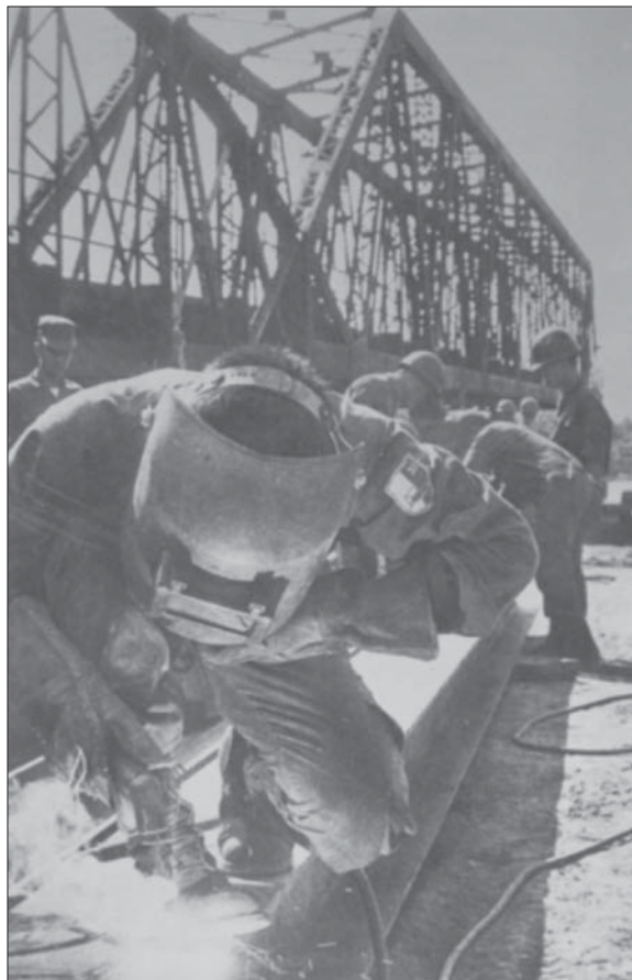
Each ARVN corps possessed a three-battalion engineer group; here a welder of 30 Engineer Bn prepares a beam for the erection of a new bridge as part of the effort to rebuild and reopen the country's highway system. (The French-built railroads had essentially been destroyed by 1962, but lengthy stretches of track also began to be reopened in 1969.) Note the welder's left shoulder patch; engineer battalions all wore halved white-and-red shields, with a black bulldozer in silhouette and a number at top right, basically similar to the design of the artillery battalion patch, which bore a cannon silhouette instead. (Nguyen Ngoc Hanh)
