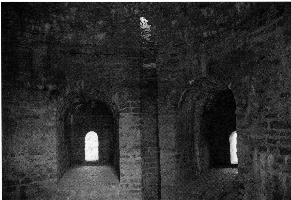
Loopholes inside the Namestnik (vicegerent) Tower of Ivangorod Fortress. Note the flue in the centre between the embrasures.
