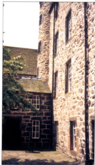
ABOVE Provost Skene's House, Aberdeen: the entrance. The original tower house is on the right and would have been entered from a door at the foot of the stair tower. Both of the projecting jambs date from 1626 or later.
