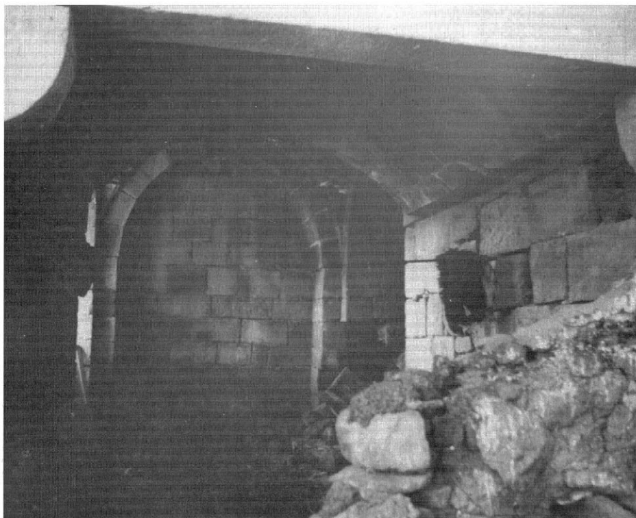
The main entrance to the early 16th century Ottoman fort at Muzayrib in southern Syria. A chain of 25 such fortifications protected the Pilgrim road from Damascus to Mecca, each being garrisoned by a small unit of Janissaries or other provincial infantry. (Author's photograph)
