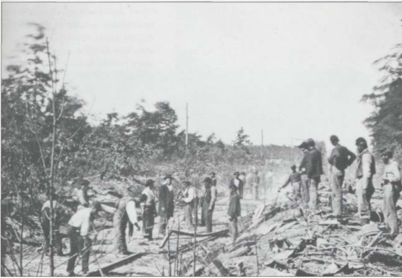
Union soldiers put aside their weapons and pick up tools to repair the damage done by Stuart's raiders. NA
