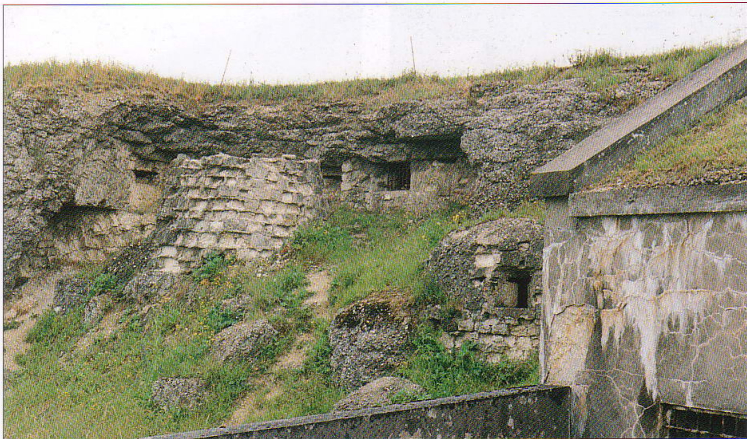
TOP Loopholes defended by machine guns at the south-east corner of Fort Douaumont. Part of the wall collapsed at this point after a direct hit from a super-heavy howitzer. (Author's Collection)
