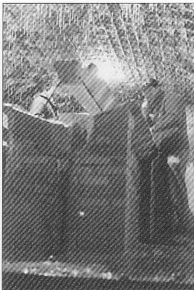
ABOVE The washing-area has sprouted stalactites during the long years Douaumont was sealed up. The facilities were Spartan by comparison with the later Maginot Line forts. (Author's Collection)
