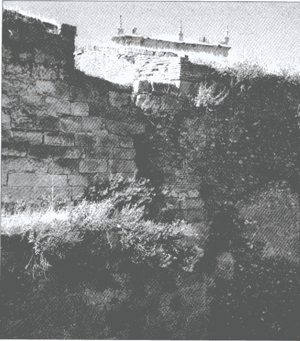
The site of the Lesser Breach at Ciudad Rodrigo. This picture was taken in 1994, before restoration work took place, and clearly shows how poor a state the wall was in. In 1812, a tower stood here before it collapsed after being shelled by British artillery. Robert Craufurd lies buried beneath this wall.
