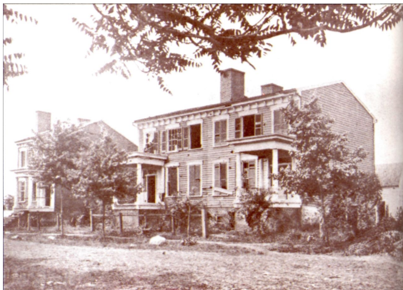
Some houses were blown up, others lost roofs or walls. Some appear almost unharmed except for the round holes left by solid shot, giving them the appearance of having been attacked by gigantic boring beetles. Judging from the entry holes, this house faces east. Exit holes are larger and more ragged.
