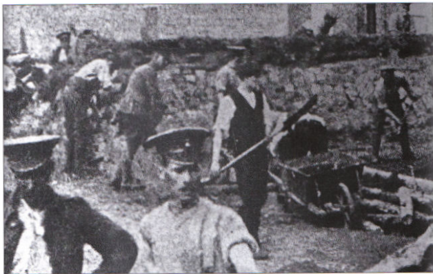
BELOW The 1st Northumberland Fusiliers building a barricade across the road from Mons to Jemappes. Note the members of the local population who not only gave tools to the British soldiers but joined in to help build the defences. This picture was taken on the morning of 23 August 1914. (Mons Museum)
