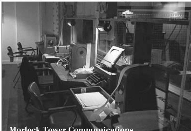
Morlock Tower Communications
